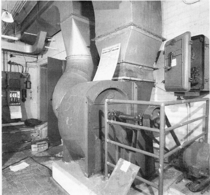
Air conditioning plant room in the Regional War Room/Group Headquarters
